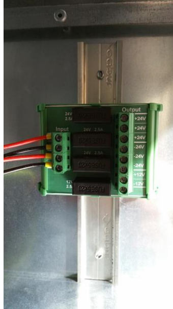
Figure 14 – Supply terminals for the distribution of the auxiliary voltages. The NEGATIVE poles must be equipped with a 2.5A fuse
