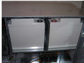
Figure 3 - 24 Vdc monoblocs series installation
