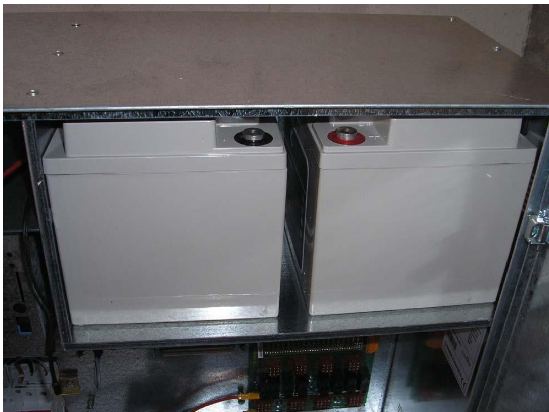
Fig. 3 - Installation of 24 V battery on board of UP
