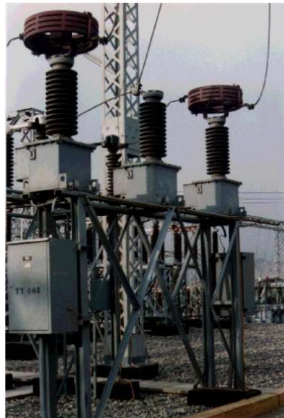
Figure 2CO (Line Trap)
